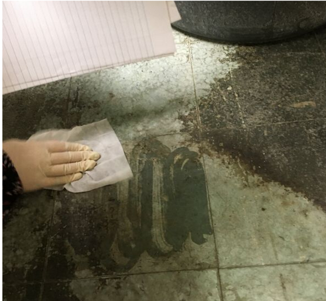
Staffer tests for lead in dust in a second-floor hallway in J. Hampton Moore School (10/25/2017)
